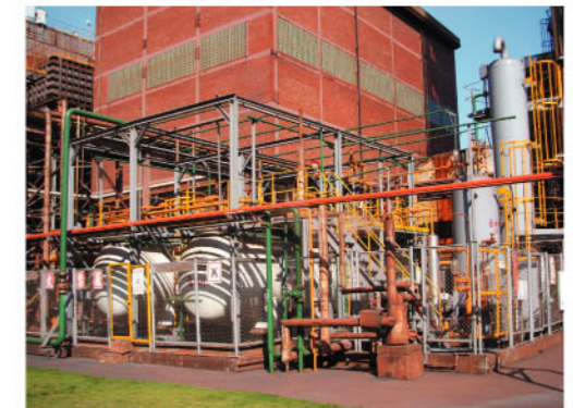
Ammonia tank of de-NO x system
