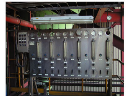
Distribution control panel of SNCR
